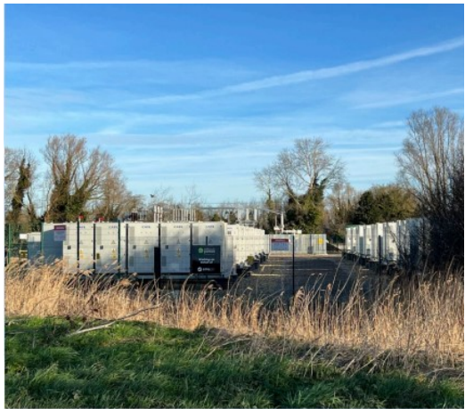
Battery Energy Storage System
